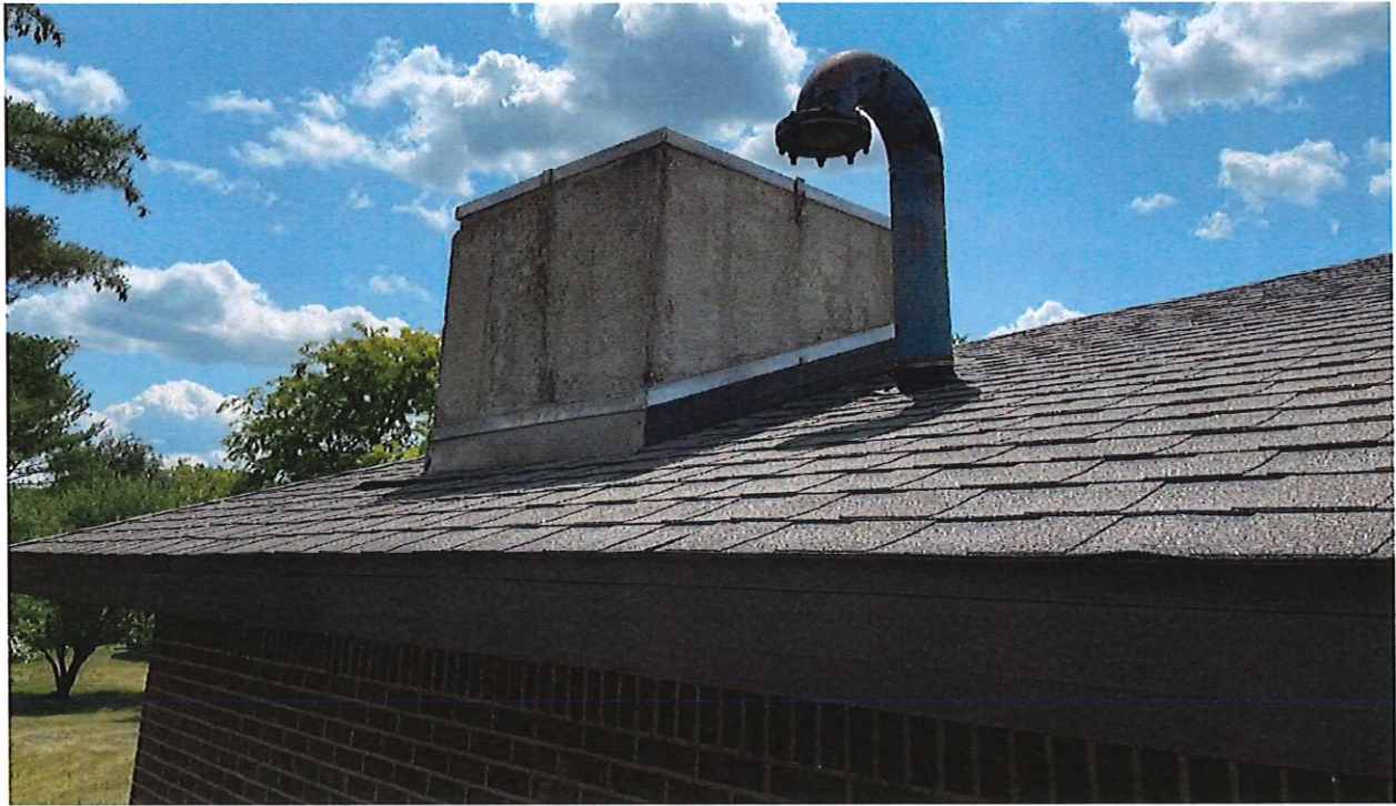
Pressure tank at Well 2 has not been in use
