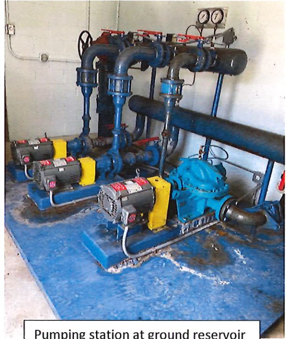
Pumping station at ground reservoir
