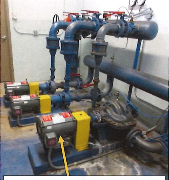
Booster pumps pressurize the system after water leaves the ground storage reservoir
